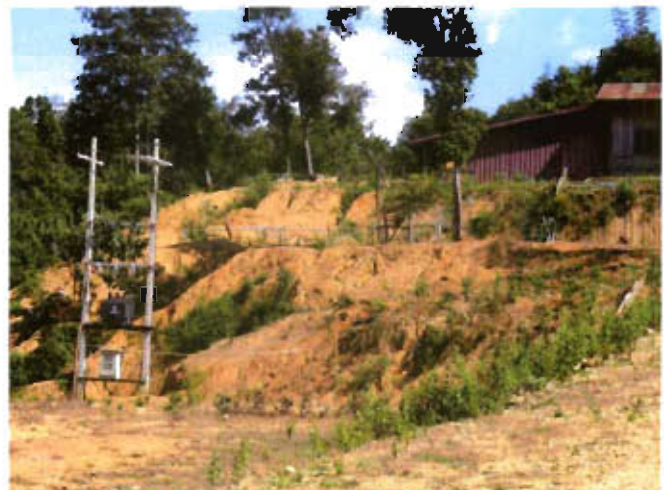
Newly installed electricity lines and temporarily unoccupied Phonesack buildings up the Nakadok valley adjacent to the NPA.
